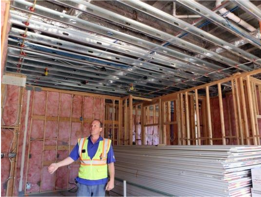
Project manager Robert Lodes talks about the apartments under construction in the former Reader's Digest building at Chappaqua Crossing in New Castle July 3, 2017. (Photo: Tania Savayan/The Journal News)
